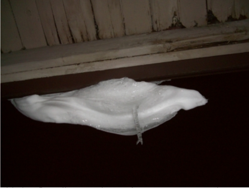
This ice floe clings to the roof over my rear porch.
